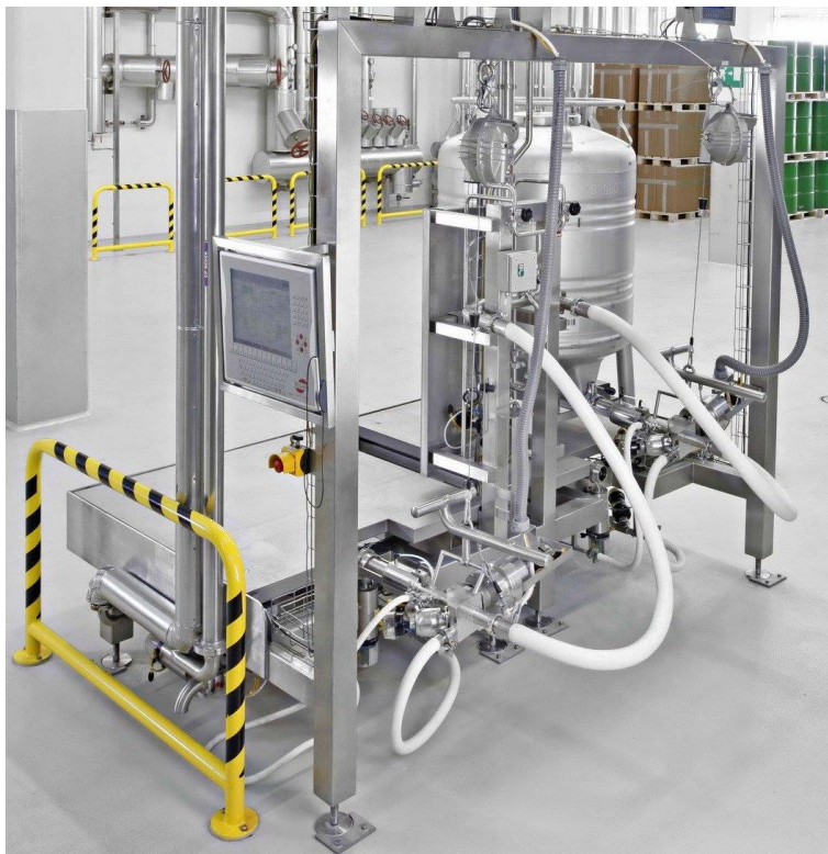
Container station with stainless steel tank, preparation for filling
